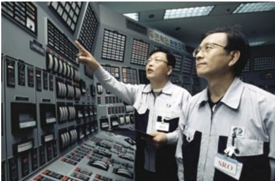
Main Control Room where real-time data is a vital part of decision-making and operations.
